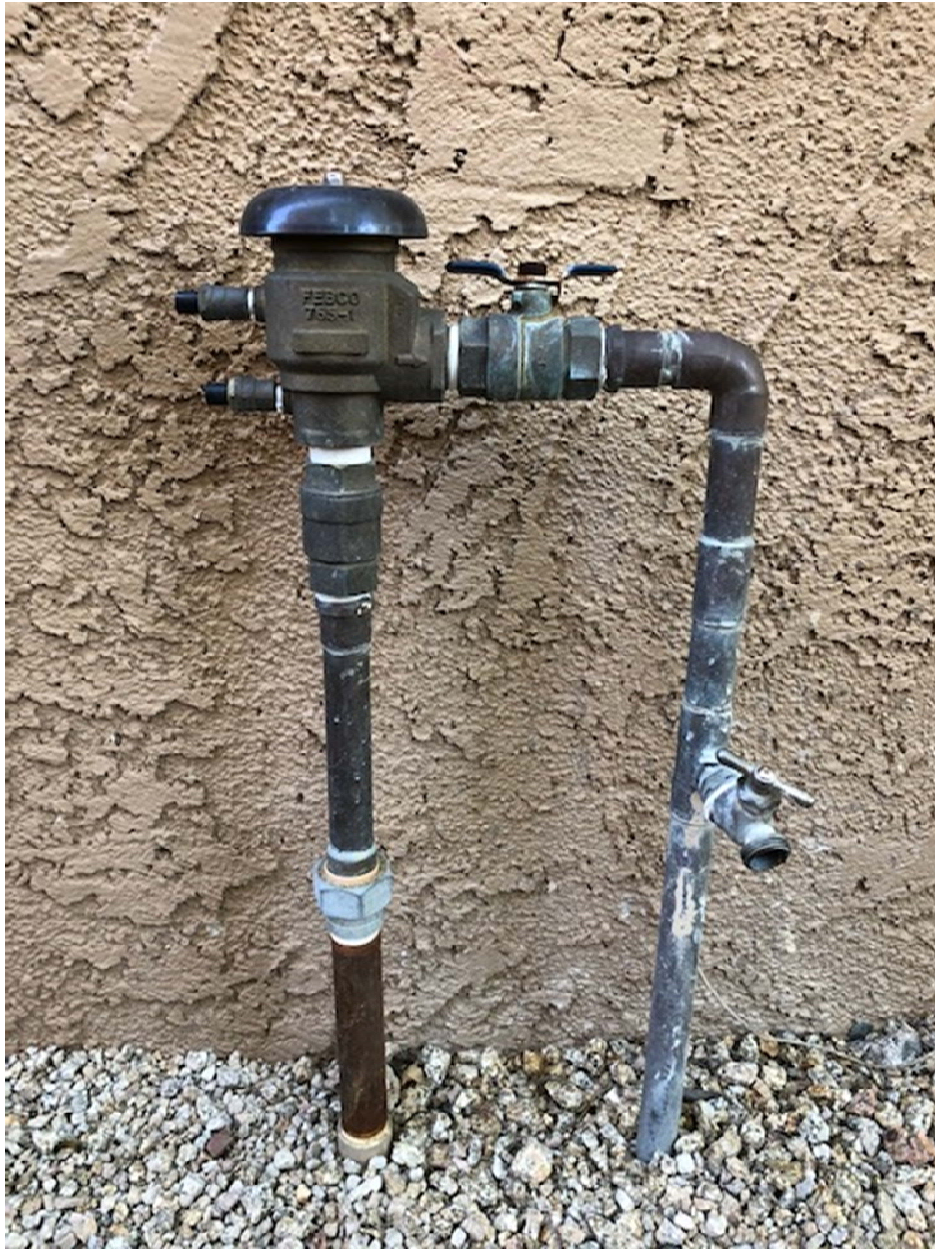
Picture 3of3. Back flow preventer #1, East side of Unit 303
