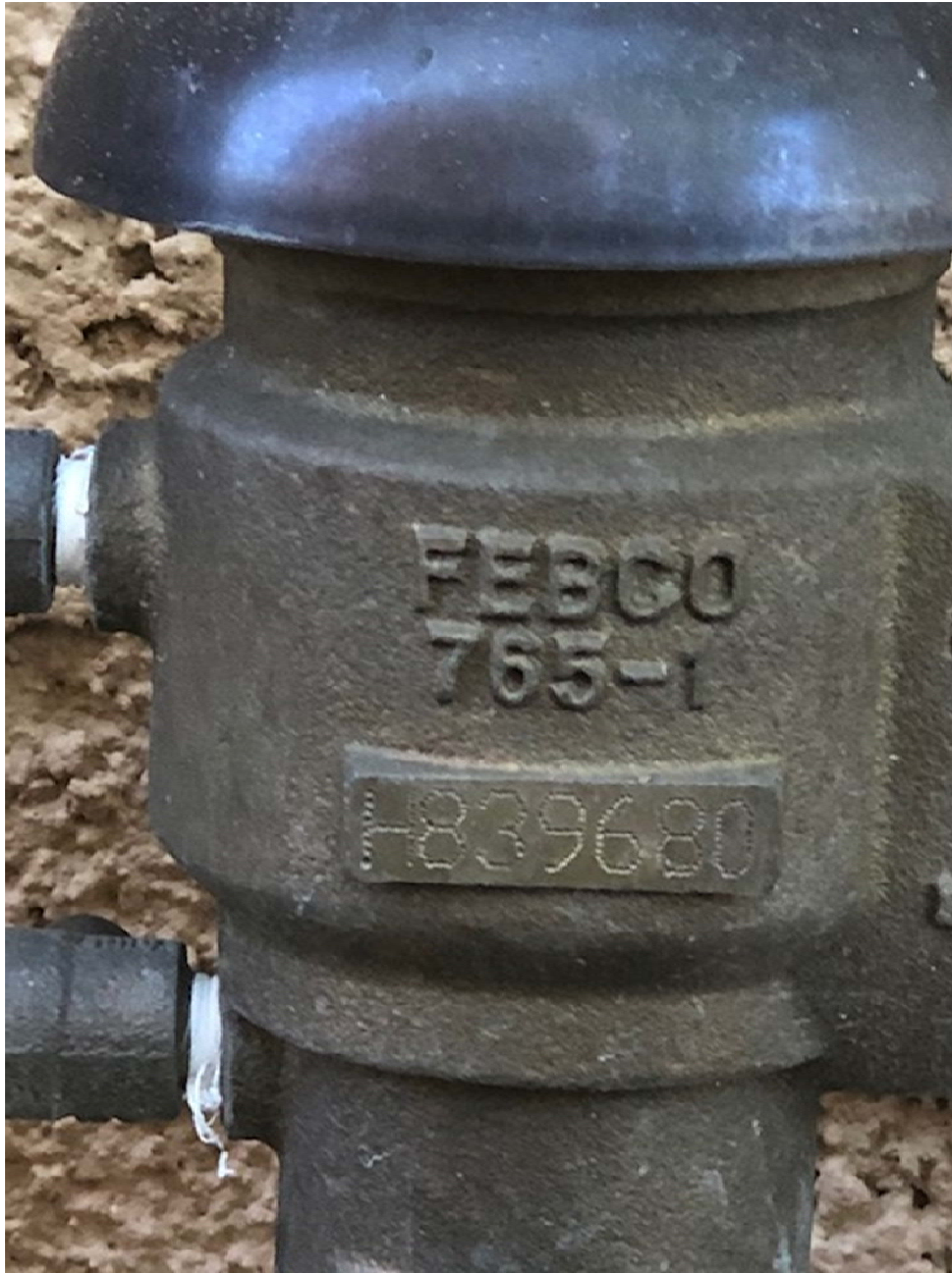
Picture 2of3. Back flow preventer #1, East side of Unit 303
