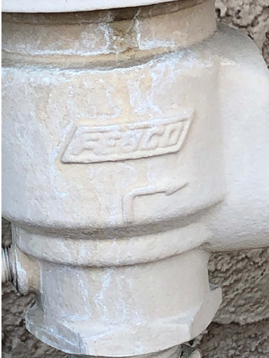
Picture 2of2. Back flow Preventer #3, South side of unit 201
